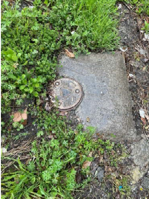
B-97 – Installed locking bar.
