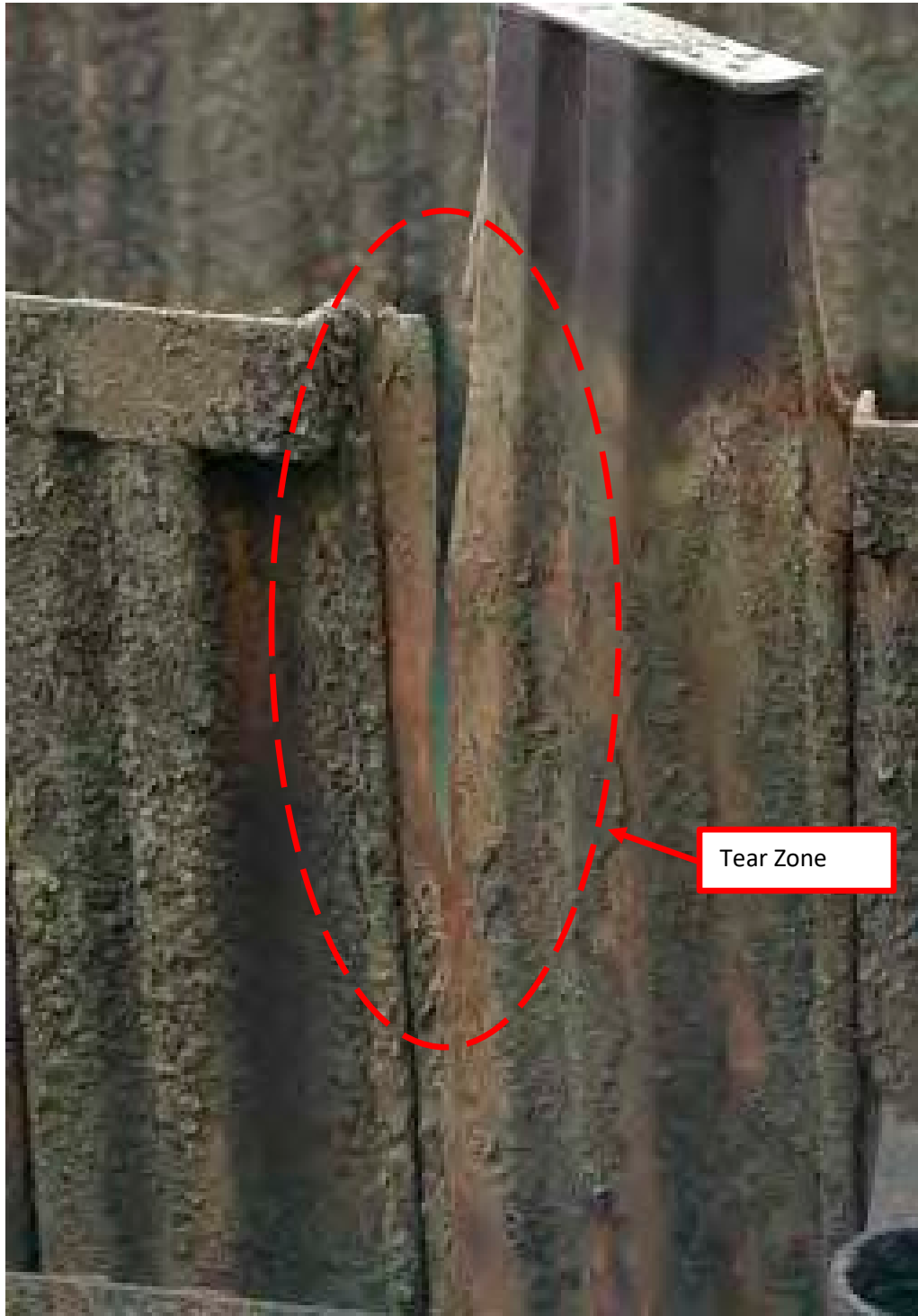
Figure 212. Sheet Piling Tear
