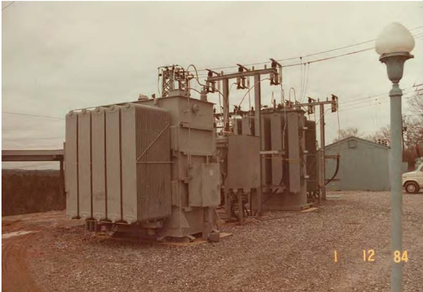
Figure 207. Relocated Electrical Equipment
