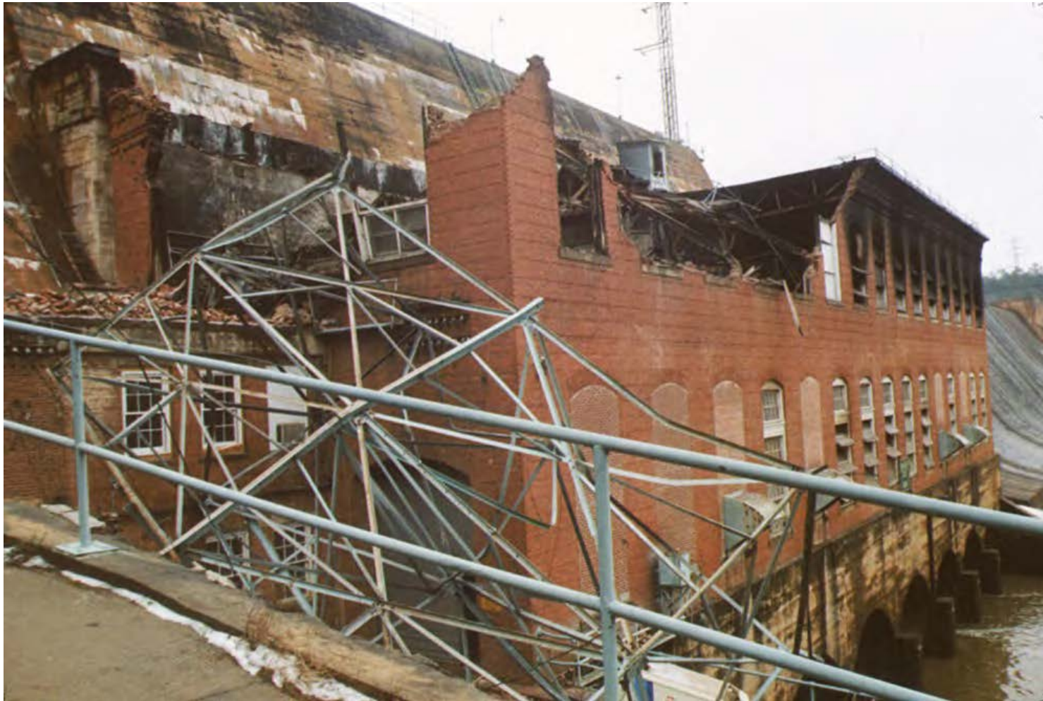
Figure 203. January 1983 Powerhouse Fire Damage
