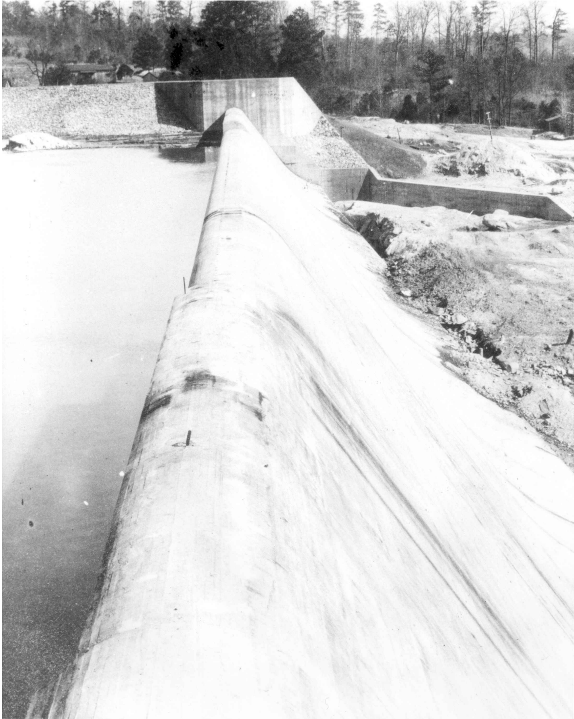
Figure 174. Spillway Crest Conditions
