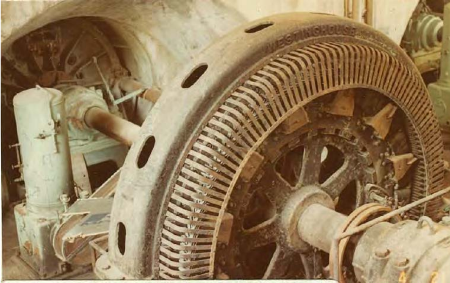
Figure 204. Fire Damaged Unit 6 Generator
