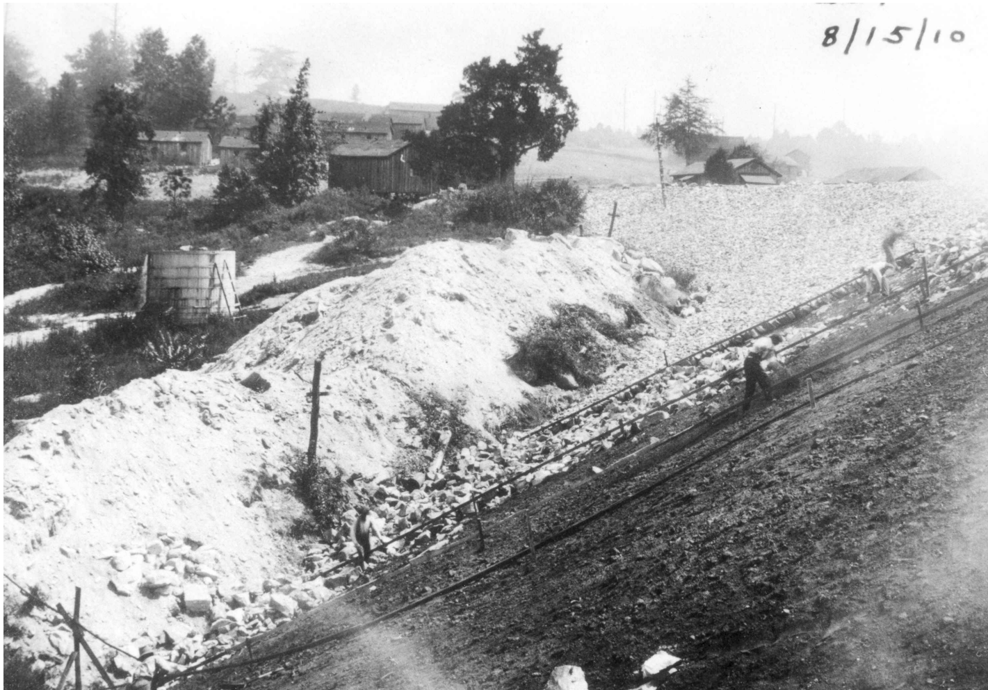
Figure 147. East Embankment Upstream Slope Rip Rapping
