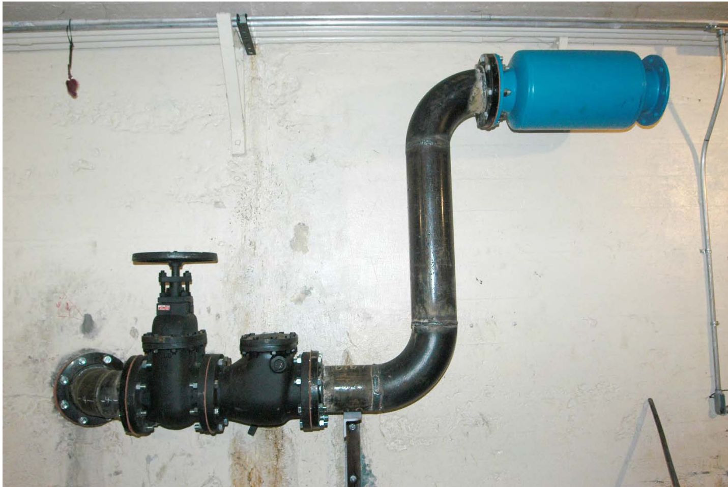
Figure 227. External Aeration Equipment
