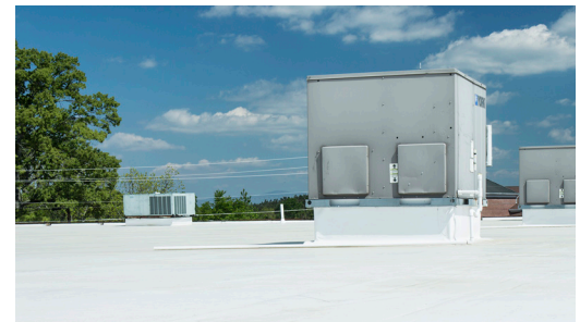
Reflective roofing systems like the one installed at the Cornelia store help keep the building cooler during the hot summer months.
