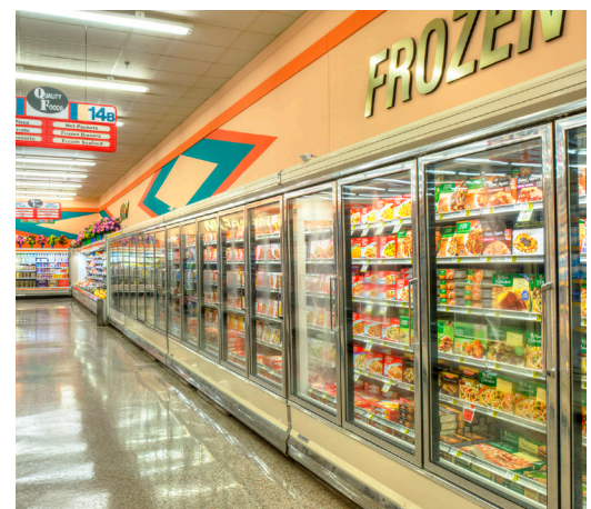
Quality Foods retrofitted its refrigerated display cases with LEDs.
