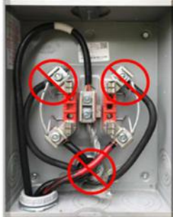
Improper routing of wires in the meter compartment, which does not allow proper clearance around the socket
