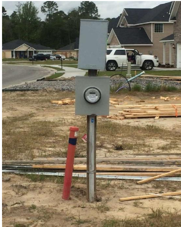
4.2 UD Temporary Service Installation
