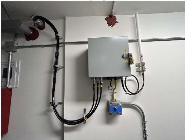
3.6 Typical Install of AMI equipment in Meter Room
