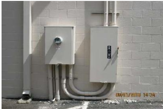
12.0 401-600 Amp, 3-Phase Transocket, Maximo# 431411
