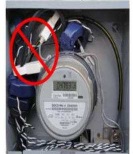
Customer owned CT meters and instrument transformers
