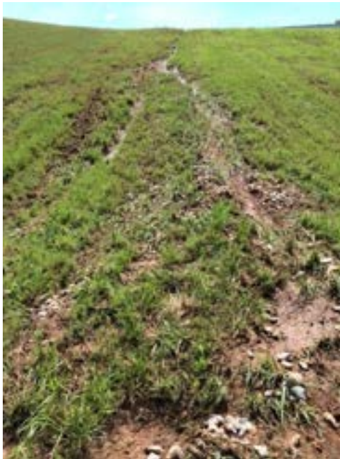
Exhibit 2 Vegetative Cover on the Embankment Northeast (Downhill) of the Return Water Pipe Rupture
