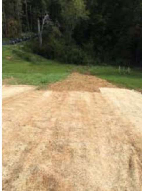
Exhibit 3 Embankment Repair Uphill from GWC-14.
