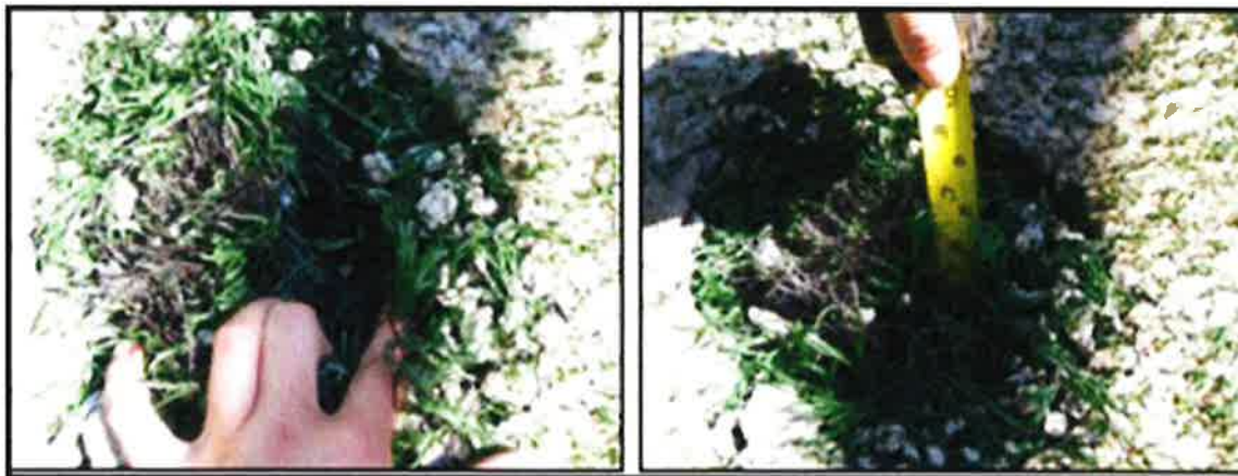
Figure 25 – Intentional Damage: Large Hole through HydroTurf®
