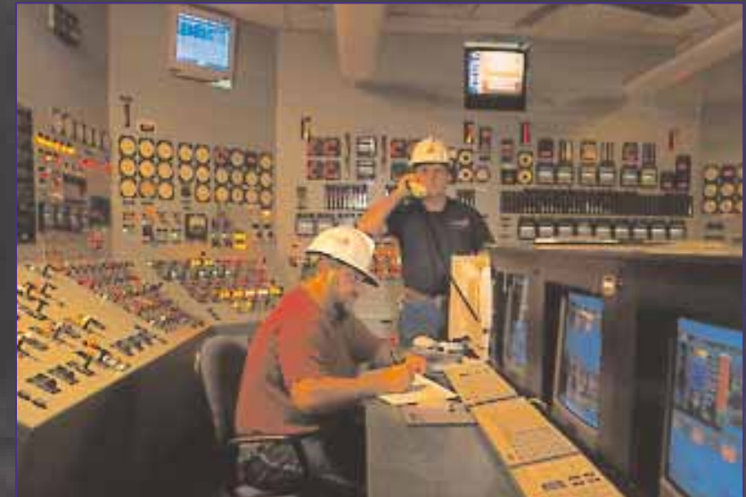
All aspects of plant operations are centrally controlled to maintain highest efficiency.
