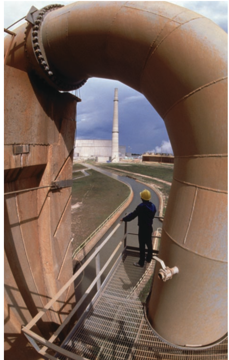
Influent pipe at one of the plant cooling towers
