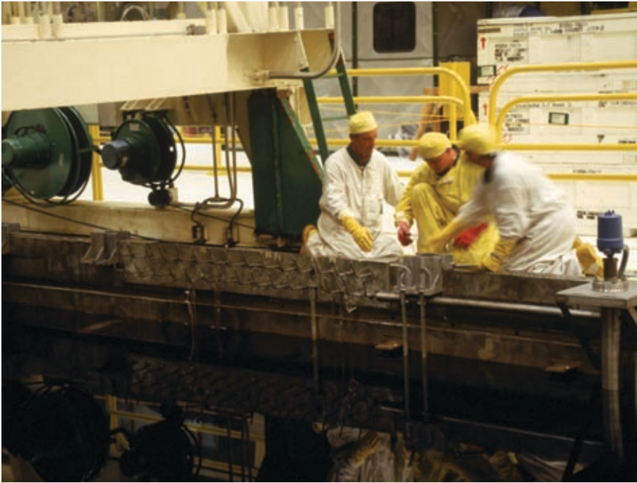
Employees working at Plant Hatch refueling floor
