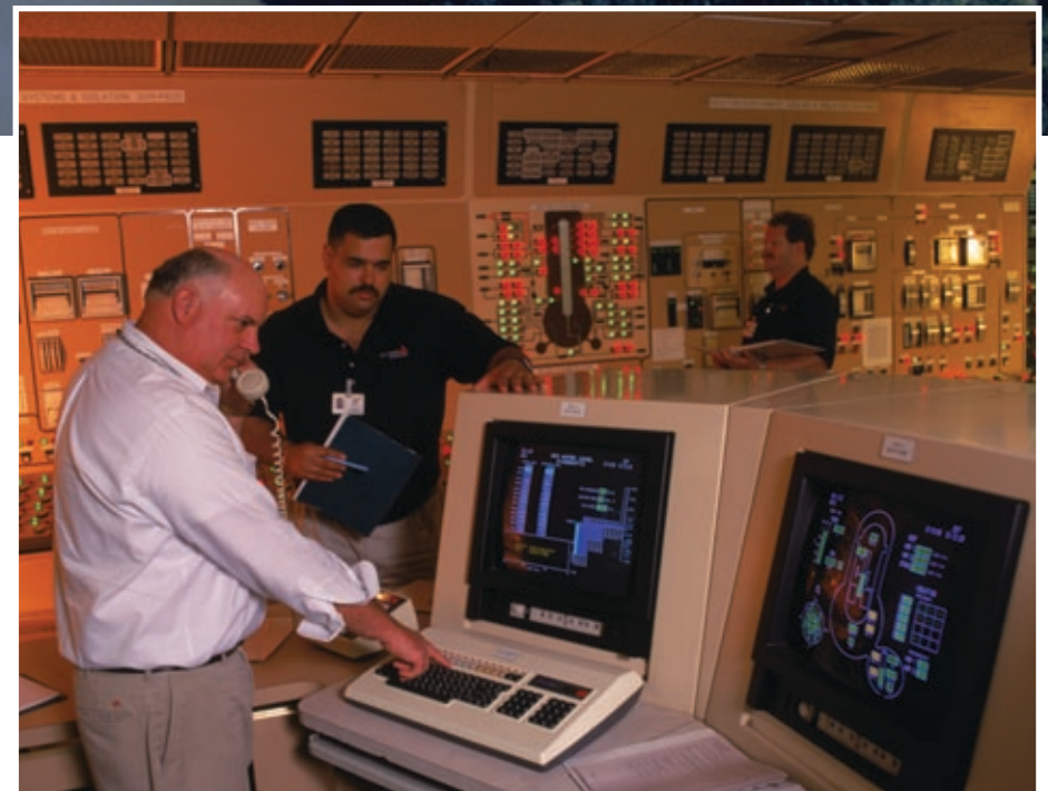
Plant Hatch control room
