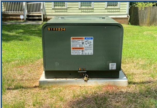
Single Phase Transformer
