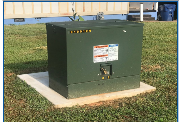
Single Phase Terminating Cabinet
