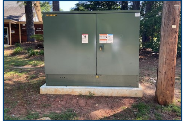
Three Phase Transformer
