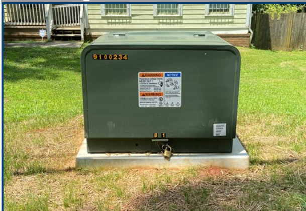
Single Phase Transformer
