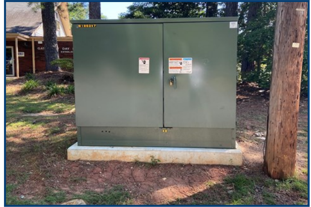
Three Phase Transformer
