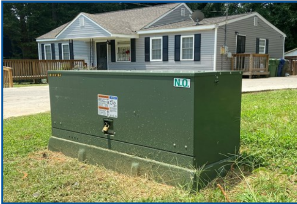
Three Phase Terminating Cabinet
