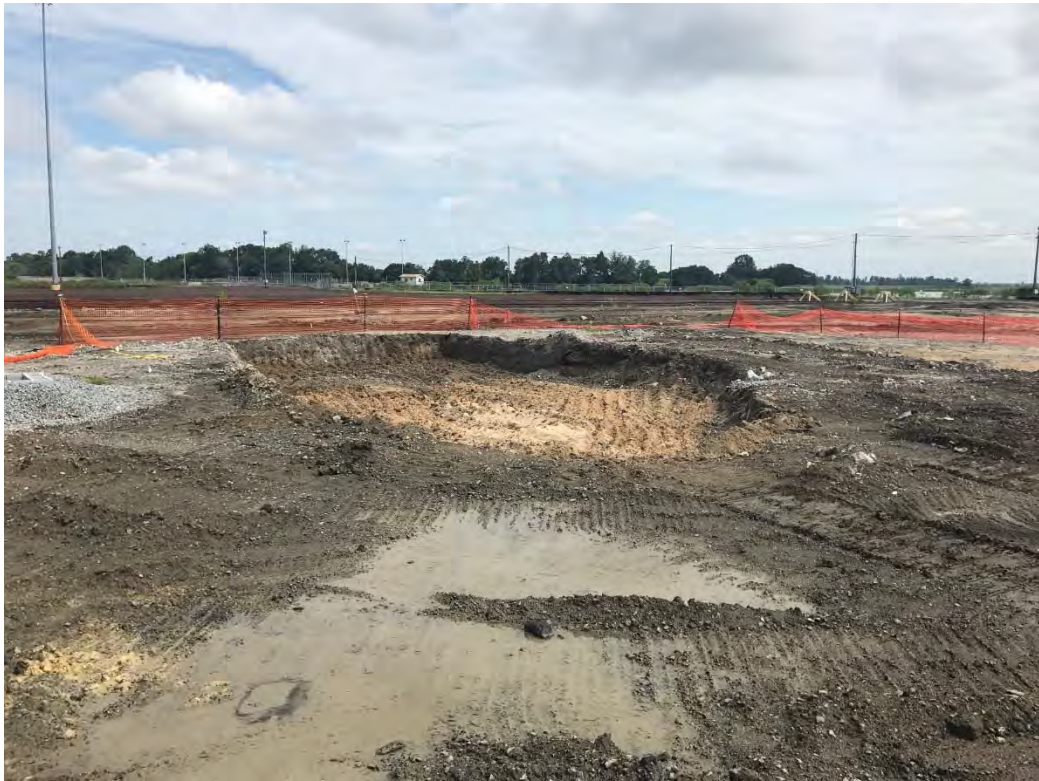
Plant Kraft Low-Voltage Switchyard
