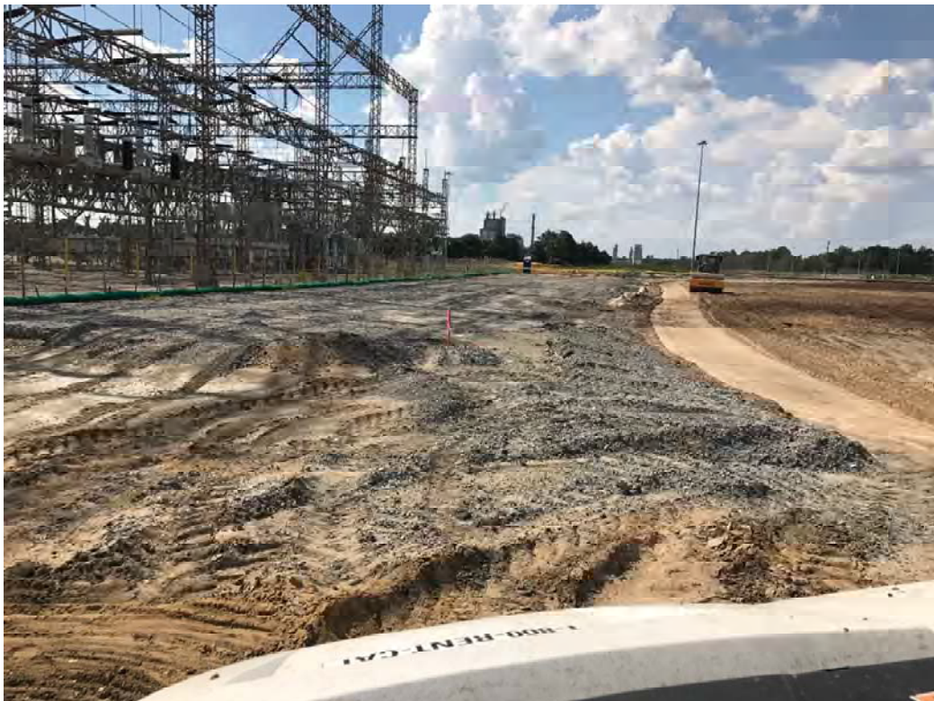
Plant Kraft Low-Voltage Switchyard
