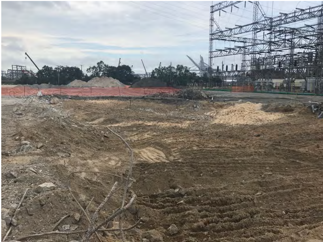
Plant Kraft Low-Voltage Switchyard
