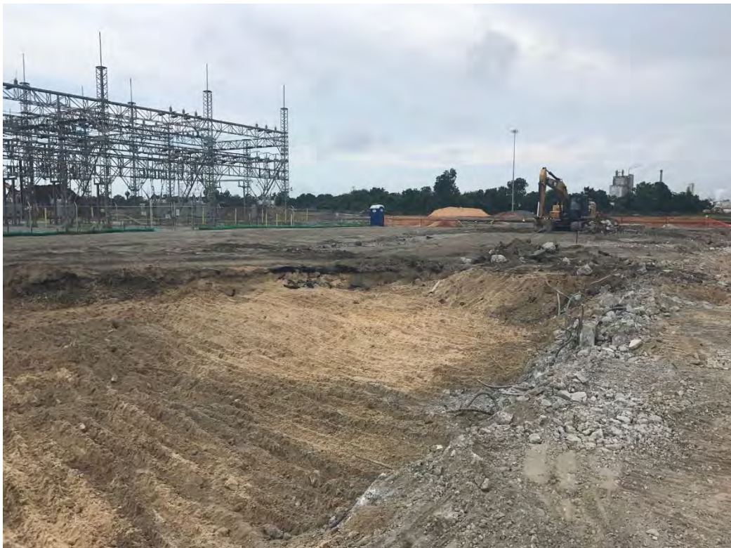
Plant Kraft Low-Voltage Switchyard
