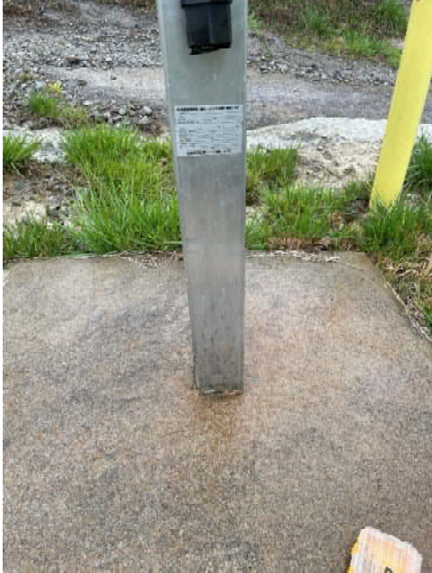
B-82 – Drilled weep hole.
