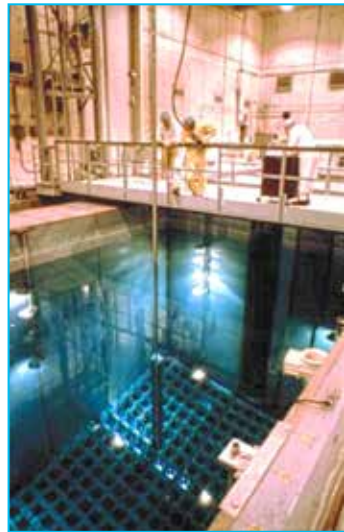
Spent Fuel Pool
