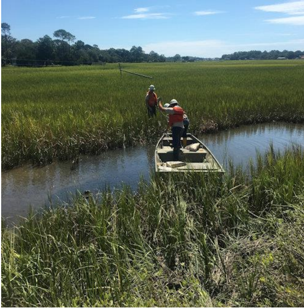
A crew from Alabama Power uses a boat to reach damaged equipment on Tybee Island.
